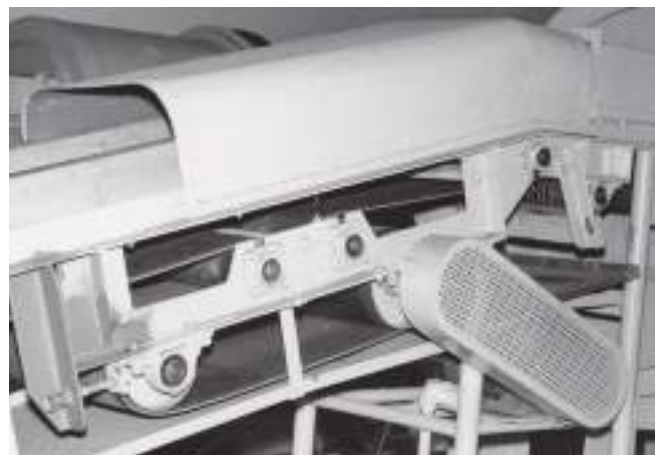
Belt conveyor driving system
